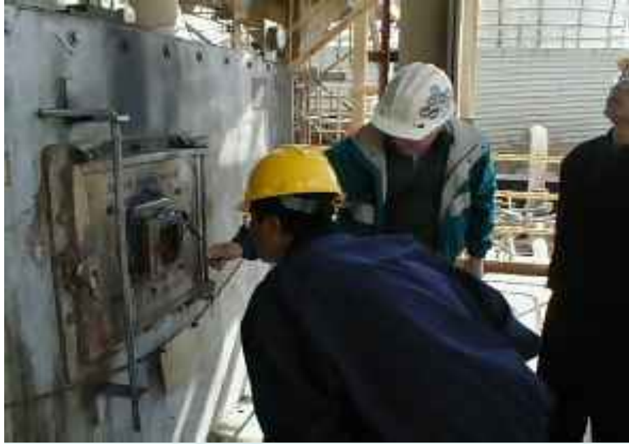
Checking out the boiler at Tracy Biomass Plant
