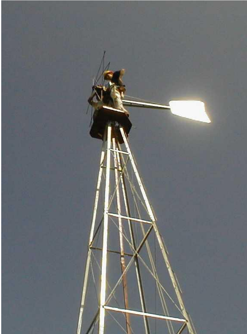
Figure 2: Water-pumping Windmill Installed by Nautilus and North Korean Engineers at Unhari in the Year 2000 10
