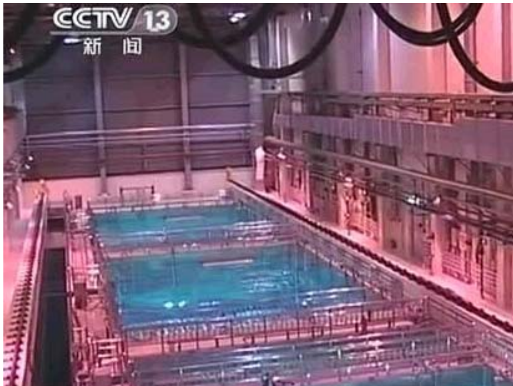
SF storage pool attached to the pilot reprocessing plant
