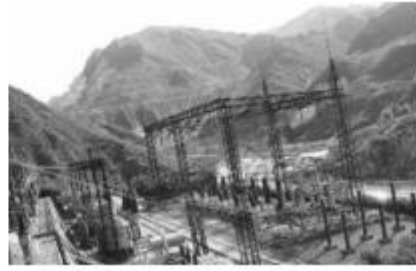
Photograph 2. The Keumgol Substation in Dancheon-si Source: South-North Korea Exchanges and Cooperation Support Association, Joint Survey Report of North Korea Mineral Resources by South-North Korea , 3rd edition, (South-North Korea Exchanges and Cooperation Support Association, 2007), 26.
