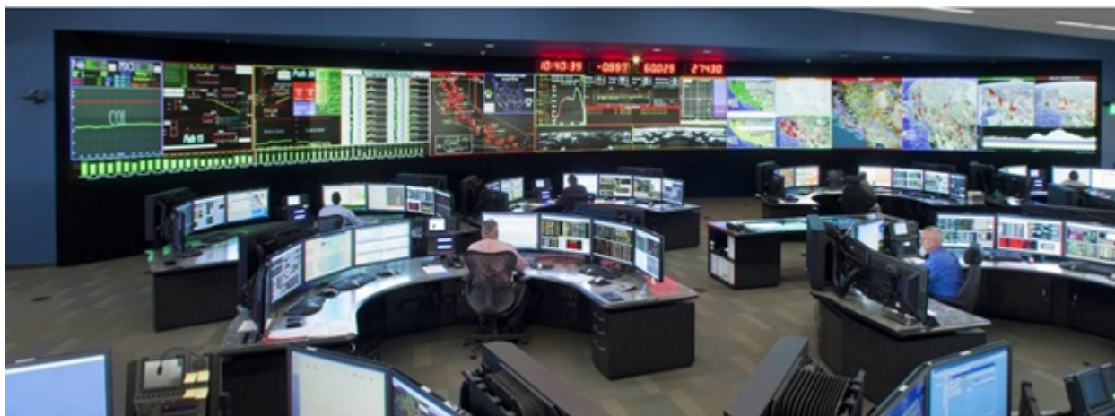
Figure 4: Control room — California ISO
