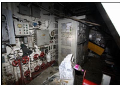
Figure 3. The Diesel Engine Room
