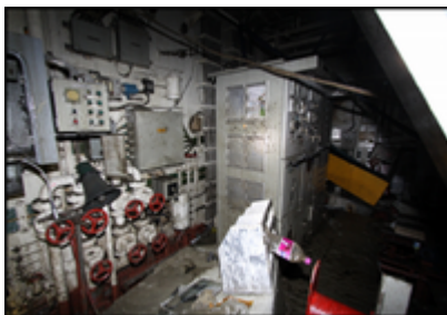
Figure 3. The Diesel Engine Room
