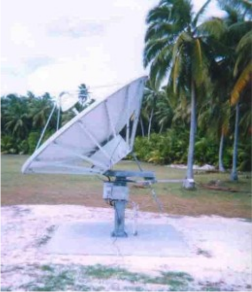
Defence satellite earth station, Cocos Islands.
