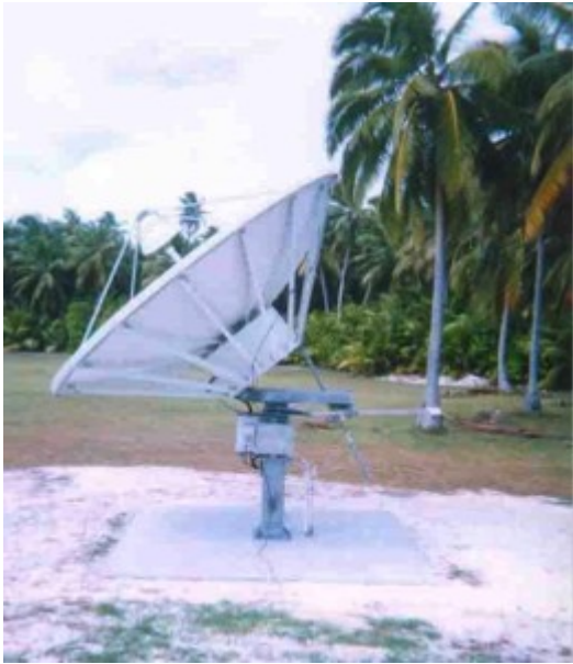
Defence satellite earth station, Cocos Islands.
