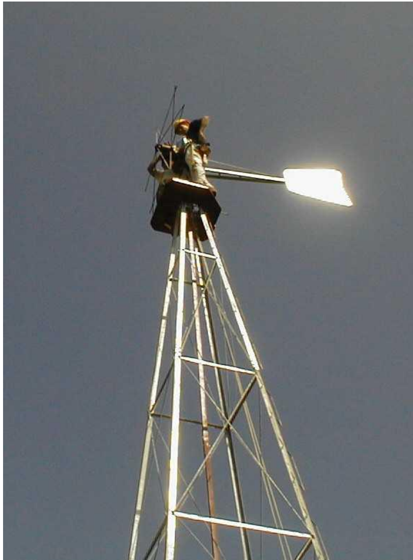
Figure 4-2: Water-pumping Windmill Installed by Nautilus and DPRK Engineers at Unhari in the Year 2000 42
