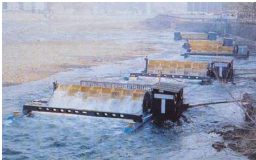
Figure 2-3: Photo of Kangae Hydro Power Plant 227
