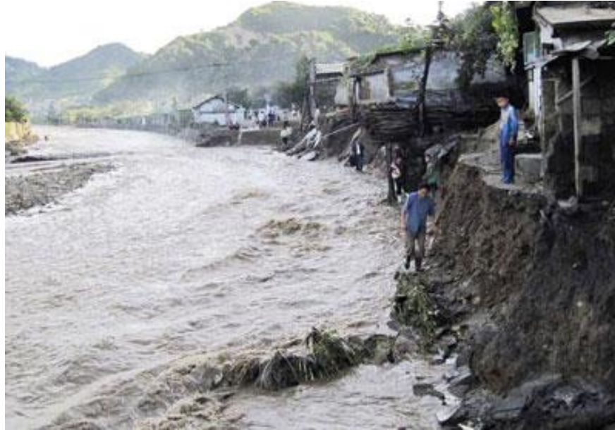
Figure 3-4: Flooding in Wonsan, DPRK in 2011 307
