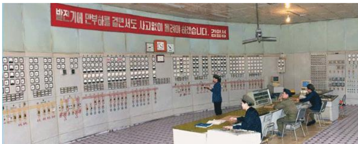
Figure 2-2: Control Room at Pukchang Thermal Power Plant 218
