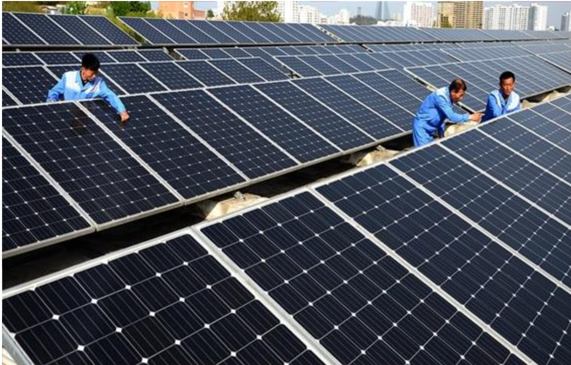
Figure 5-21: Solar PV System Installed on Ryuwon Footwear Factory in Mangyongdae District, Pyongyang (Source: Korea Friendship Association USA)
